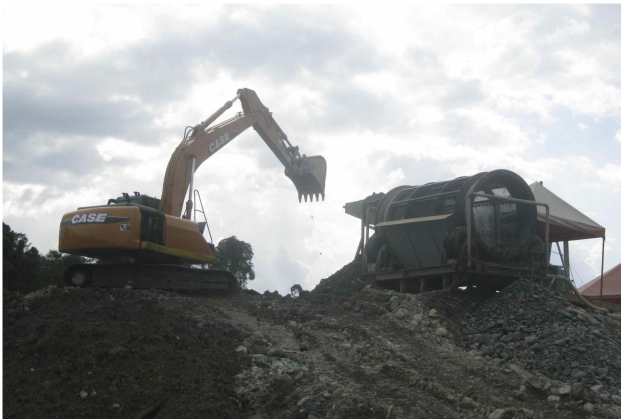
Excavator feeding process material to trommel at bulk mining operations, Martinez Mine
