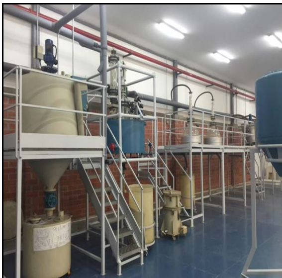
Figure 6: Gold Refining Equipment, Cali Facility
