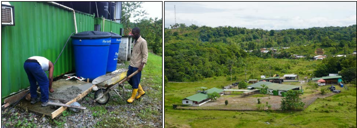
Figures 3 and 4: Adding a new platform for extra camp water storage. Novita camp/compound with helicopter pad in foreground, photo taken from Colombian Army Base located on ridges behind the camp.
